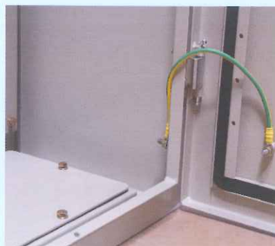
EARTHING BETWEEN BODY & DOOR
