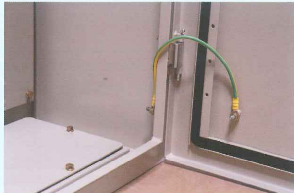
EARTHING BETWEEN BODY & DOOR
